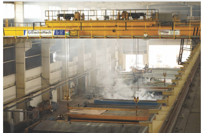
Galvanising & Pickling Area Crane
