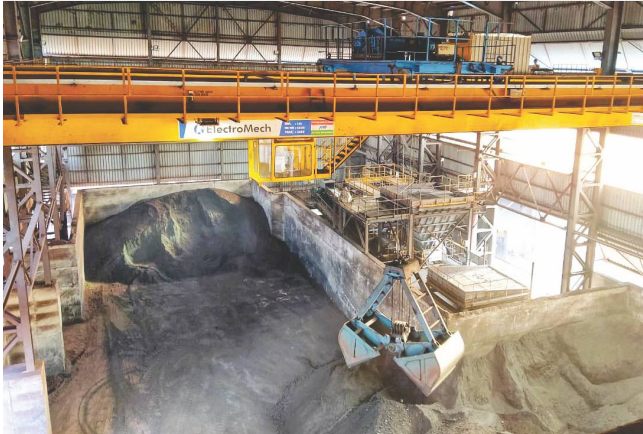
Bulk Material Handling Solution
